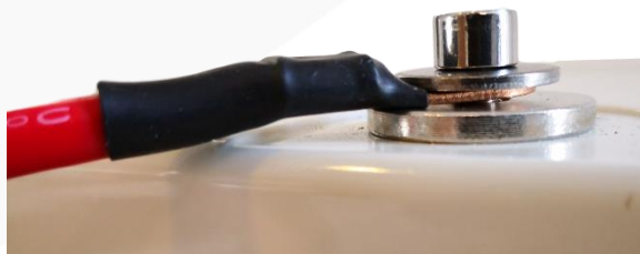
Figure 3. WRONG! Loose connection by using too long bolt
